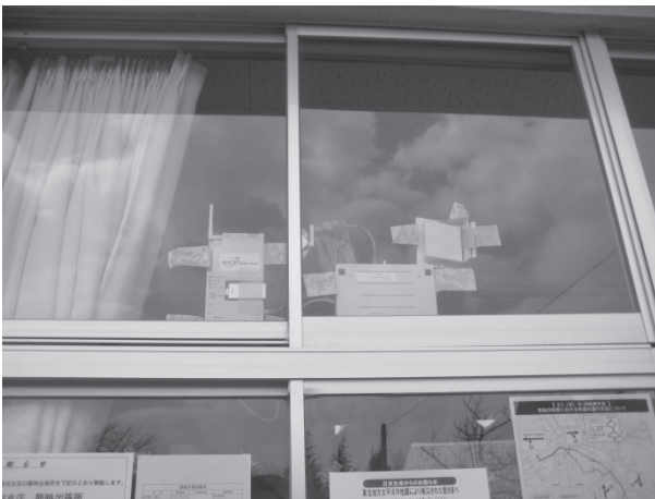
Cognitive wireless router (Left) and mesh RMR router (Right)
