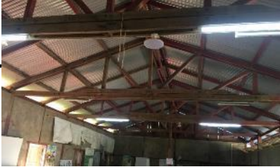
Lighting by LED lamps
